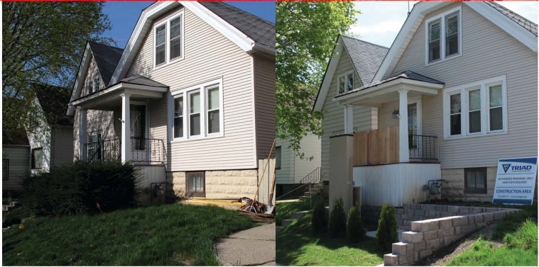
A south side Milwaukee house (left) is transformed (right) as Triad Construction Inc., West Allis, makes modifications to the home's entryway. The company installed a 6-foot lift to transport the homeowners' 4-year-old son, who uses a wheelchair, from the front porch to the sidewalk.
